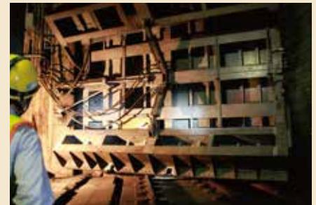
Watertight doors (in tunnels)
